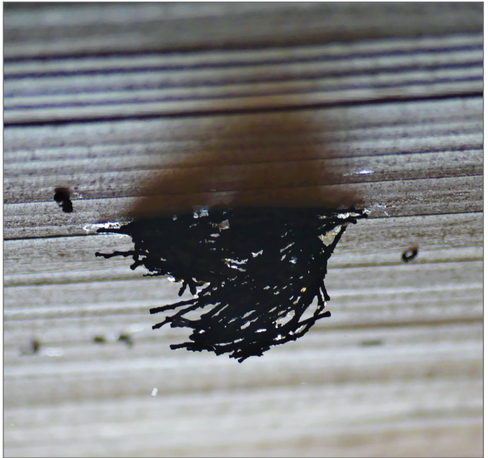
FIGURE 5: Nest on the wall of tower T4 at the Selkirk Mental Health Centre taken from underneath on 23 September 2021. Photo credit: Timothy Poole, Manitoba Government.
