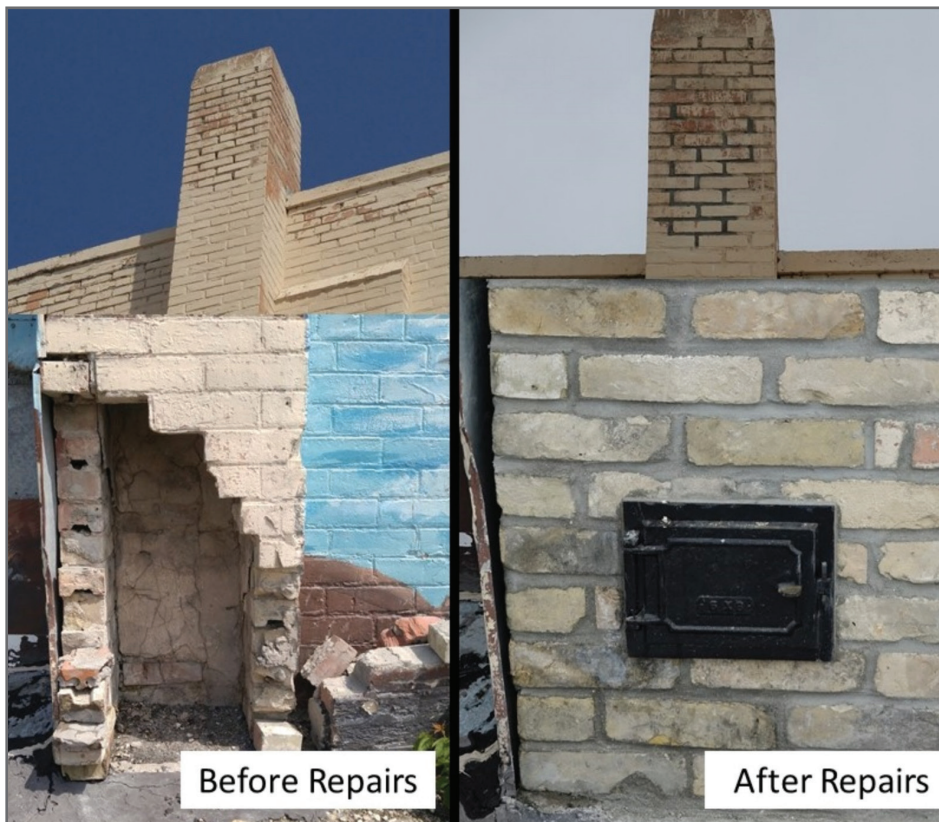
A chimney repaired at Roxy Lanes in Winnipeg. The top of the chimney required repointing while the bottom of the chimney had a large hole filled in and a clean-out installed after it was hit by a car. Photo credit: Amanda Shave.
