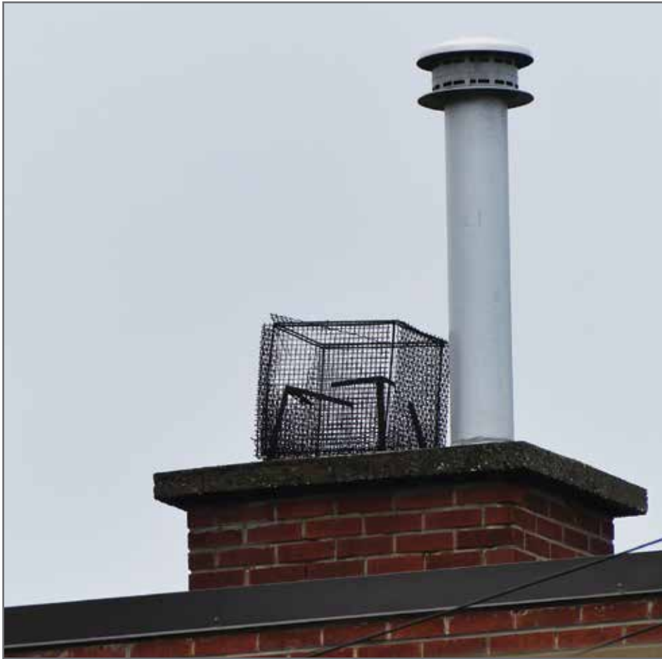
FIGURE 2. Damaged pest exclusion screen accessed by Chimney Swifts in Winnipeg. Note the spark arrestor is covering a lined flue and the exclusion cage is over an open flue. Photo credit: Timothy Poole.
