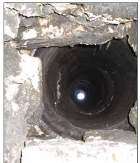
FIGURE 4. Inside of clay-lined chimney at Trinity United Church. Photo credit: Gordon Ogilvie.
