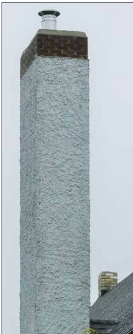
FIGURE 3. Two chimneys at St. Ann's Church, Winnipeg. The chimney in the foreground has two flues. In the foreground is an open flue, and the spark arrestor covers a closed flue. The chimney to the right is two bricks wide only. Photo credit: Timothy Poole.
