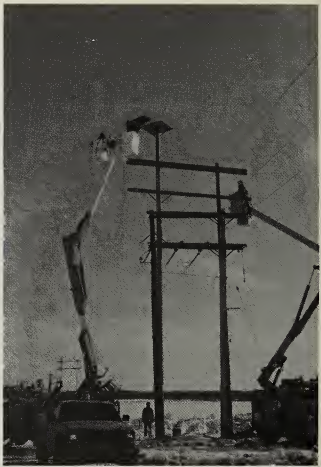
Another Manitoba Hydro crew installing a nest platform during replacement of a fire-damaged 25,000 volt structure on the shore of the Waterhen river David Vanderburgh
