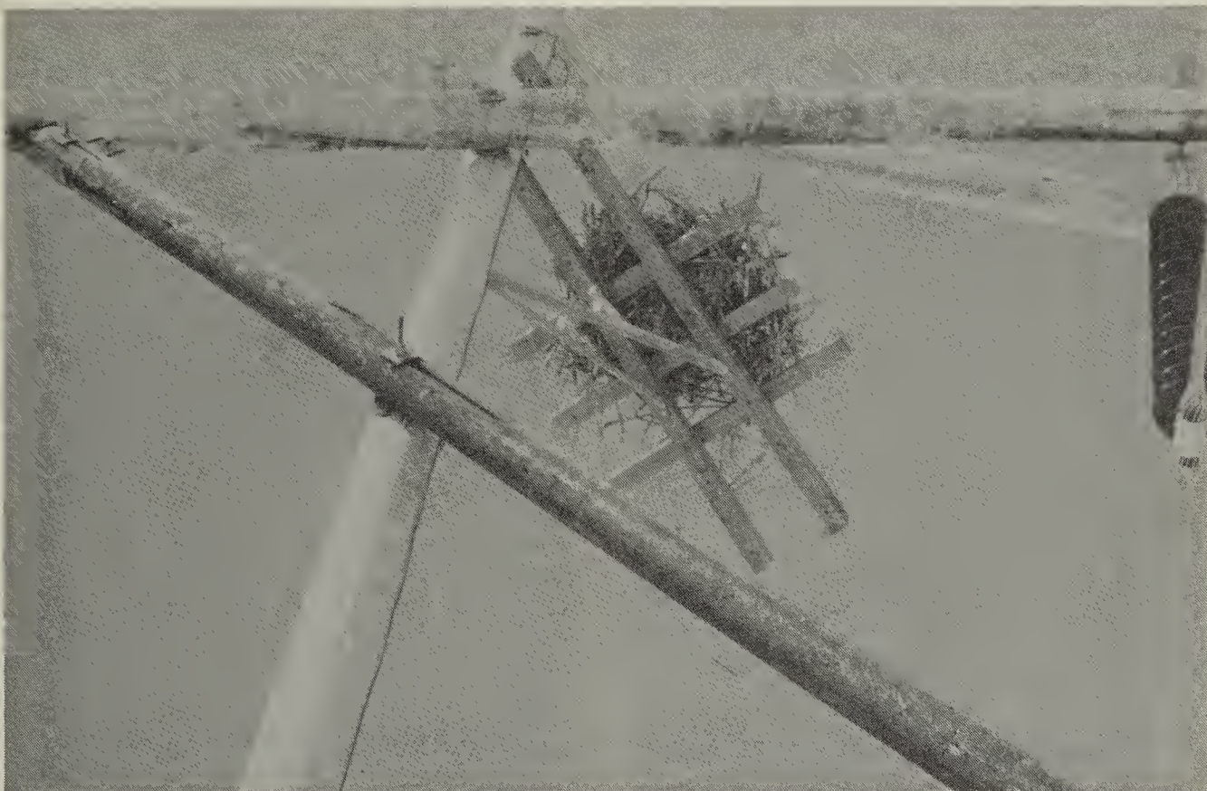
Newly installed platform c/w nest which the crew moved from the centre of the structure
