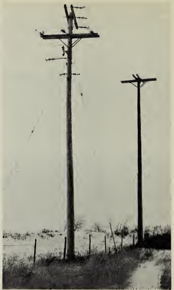
Special "nesting pole" installed to attract Ospreys away from 25,000-volt corner pole.
