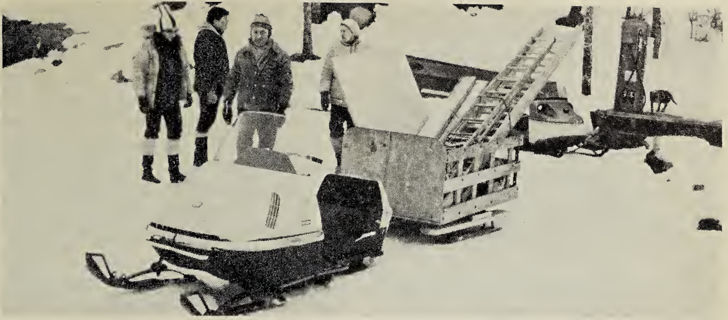
Osprey platform building crew at Loon Lake, left to right: Betty Donovan, Bruce Donovan, Frank Scott, Mary Houston.
