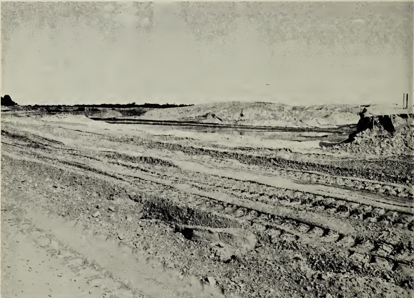
The beginning of the construction of the Ste. Scholastique 2½ mile runways which will be suitable for the jumbo jets and supersonic transports.
