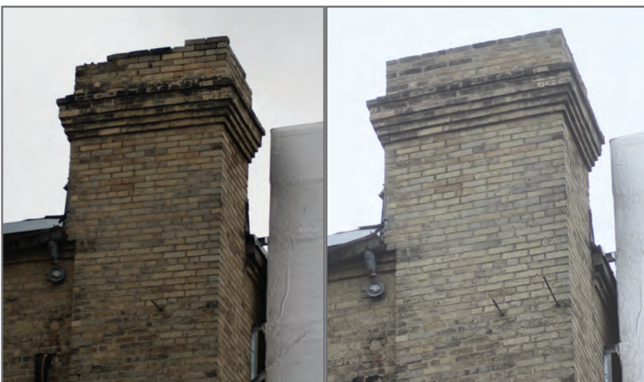
FIGURE 5. A chimney repaired in the Manitoba Chimney Swift Initiative preservation program. Before (left) lost bricks and failing joints are apparent before the repairs (right). (Photo copyright - TF Poole, 2016)
